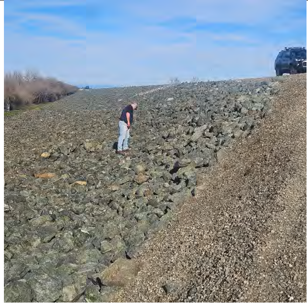
Slough along North levee (N. of I80, east of Causeway)
