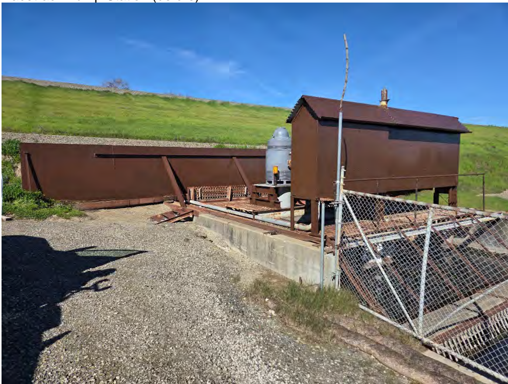
Racetrack Pump Station (after)
