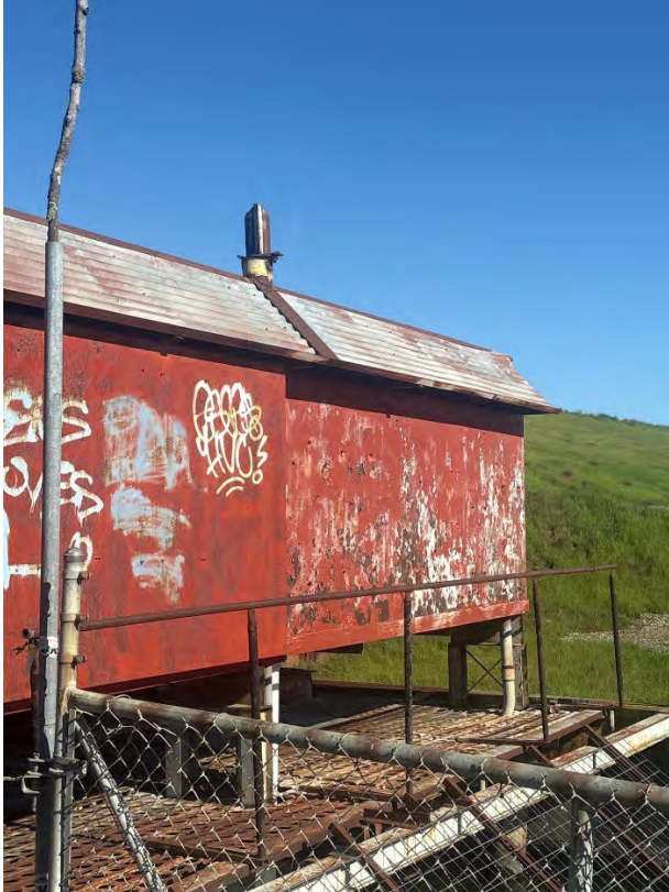
Racetrack Pump Station (before)
